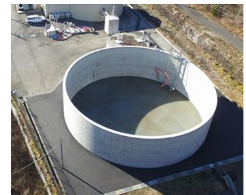
Digested liquid storage tank
